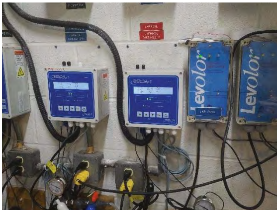
Current Control Systems
