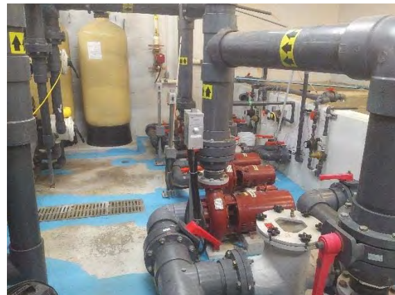
SARC Pools Mechanical Room
