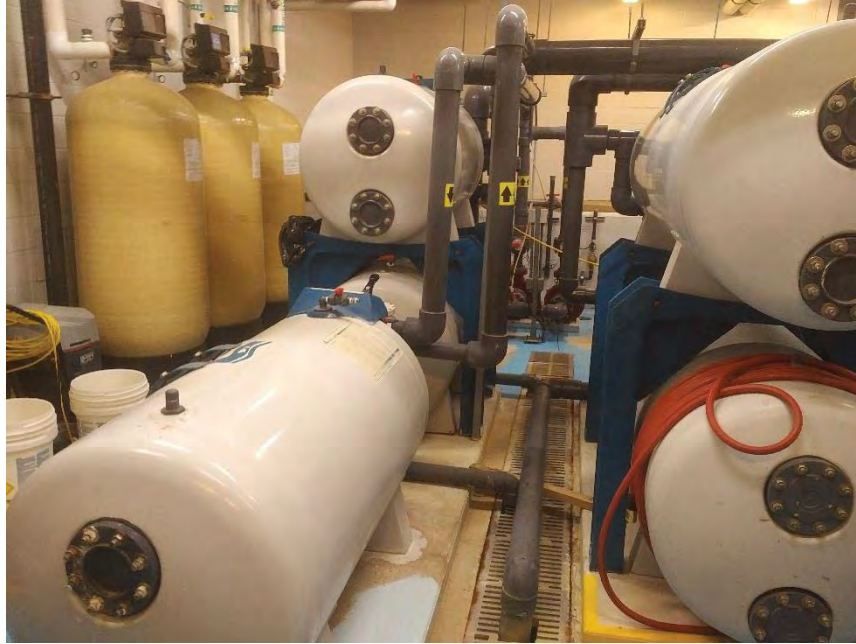
Current High Rate Sand Filters at the SARC Pools
