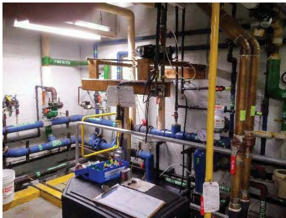
AFLC Pool Mechanical Room
