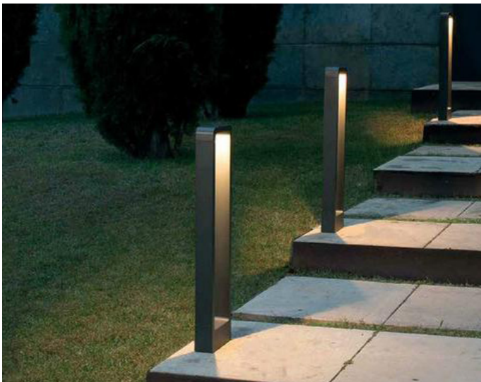
Figure 13.3 Example of energy efficient LED lighting.
