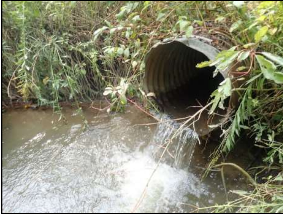
Photograph 5. Tannery Creek West Tributary – Perched Culvert (September 16, 2020)
